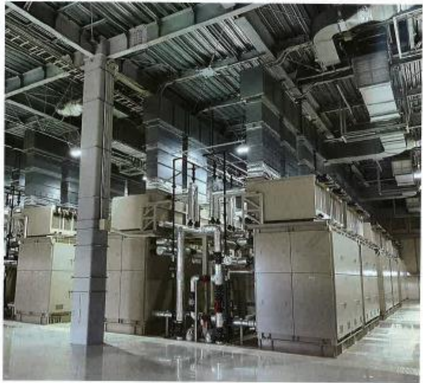
Squeaky clean: Sumitomo's 15MW/60MWh vanadium flow system in Hokkaido
